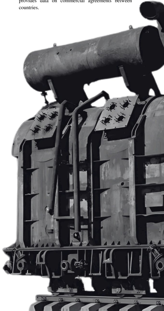
THE BATTLE FOR LIGHT™ INSTALLATION: A DESTROYED TRANSFORMER FROM UKRAINIAN THERMAL POWER PLANTS AFTER RUSSIAN ATTACKS.
